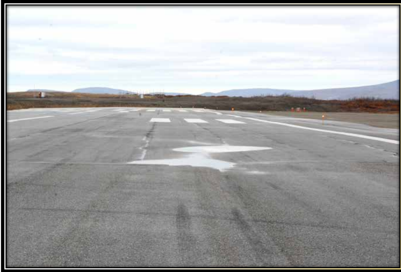
Main runway depression & ponding
