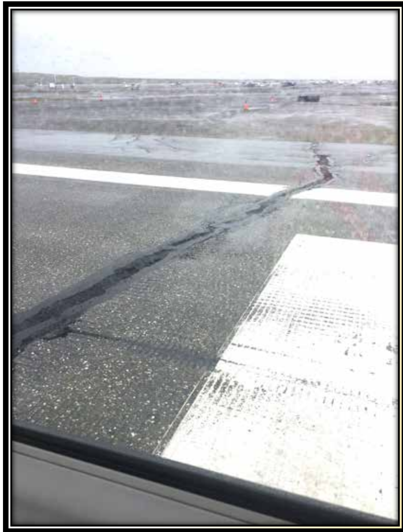
Main runway transverse crack
