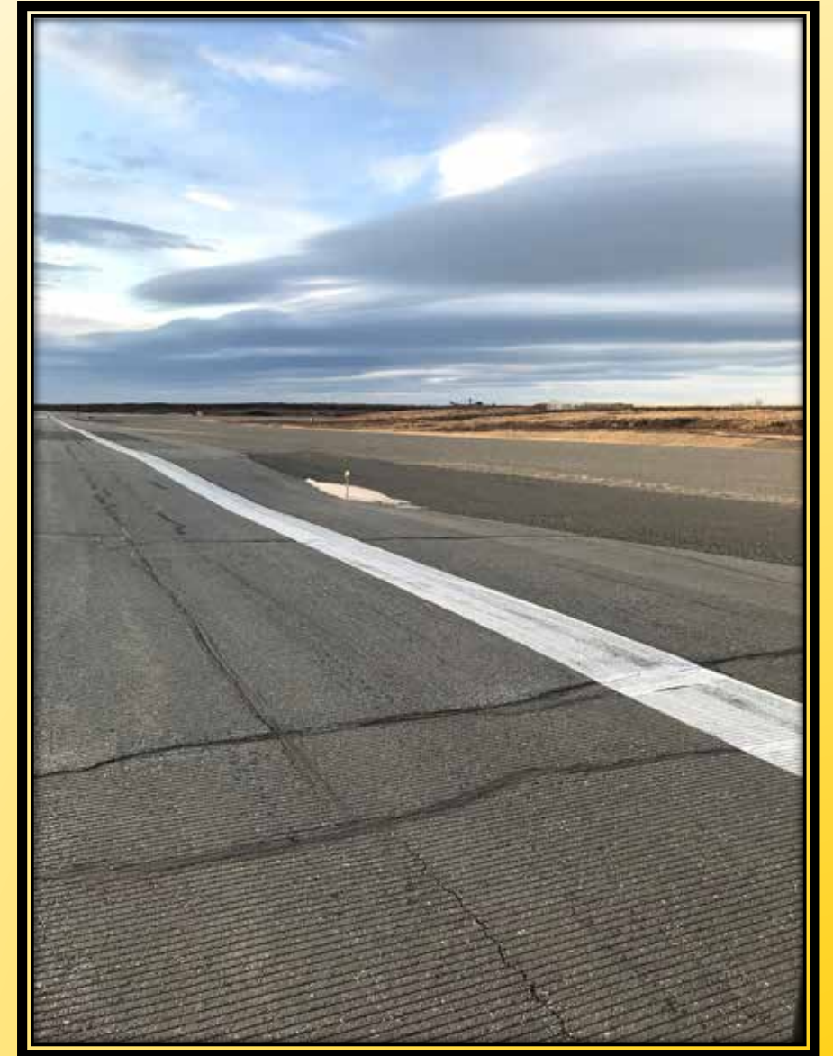
Crosswind runway dips in shoulder
