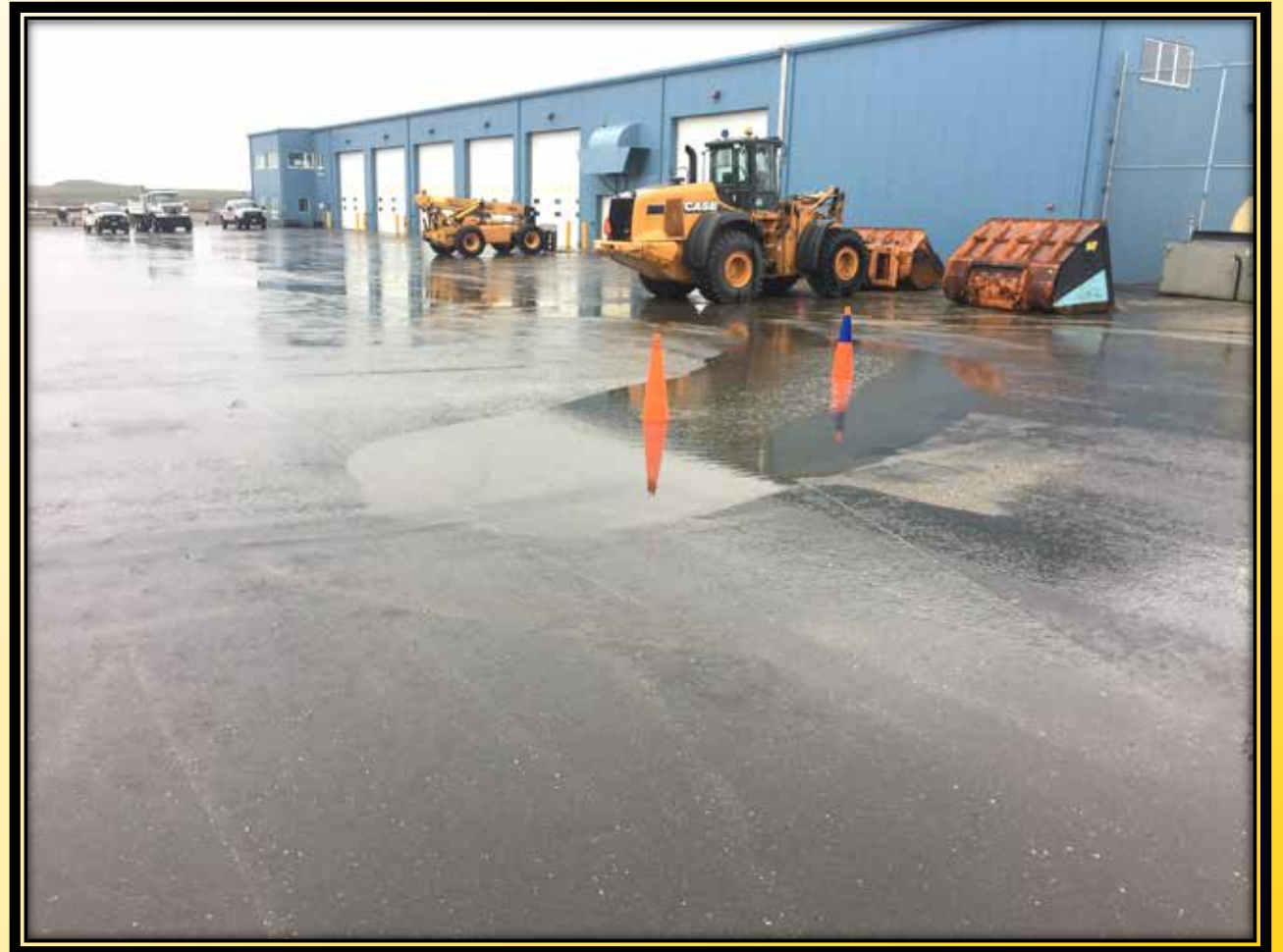
Apron depression & ponding
